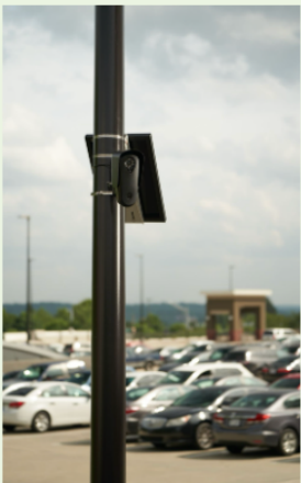
Solar & Existing Pole
